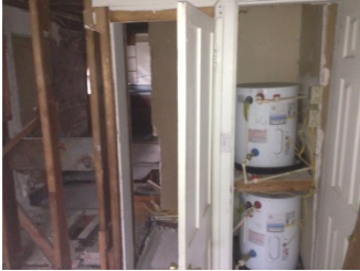
Code Correction funds were utilized to relocate a hot water heater that was illegally positioned in an apartment that was not serviced by the unit.
