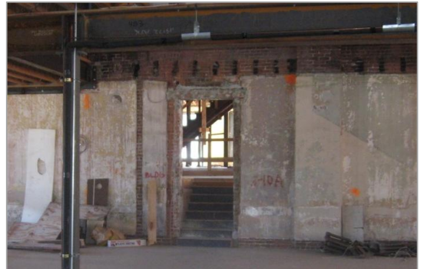
Difference in Floor Alignments between Two Consolidated Buildings
